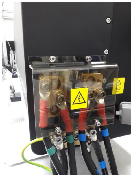
DC connections showing the plastic shield fitted
